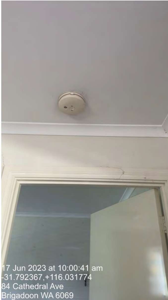
Smoke alarms were installed.
